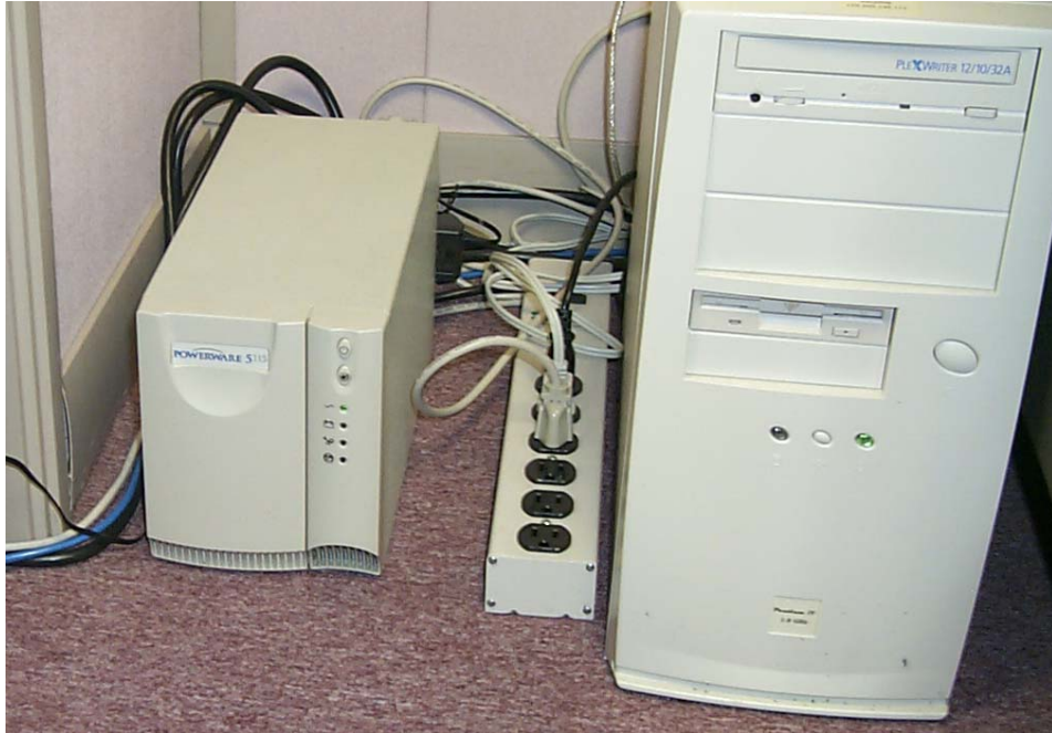
A PowerWare UPS is shown on the left and a Leviton surge-protected power strip in the middle.
